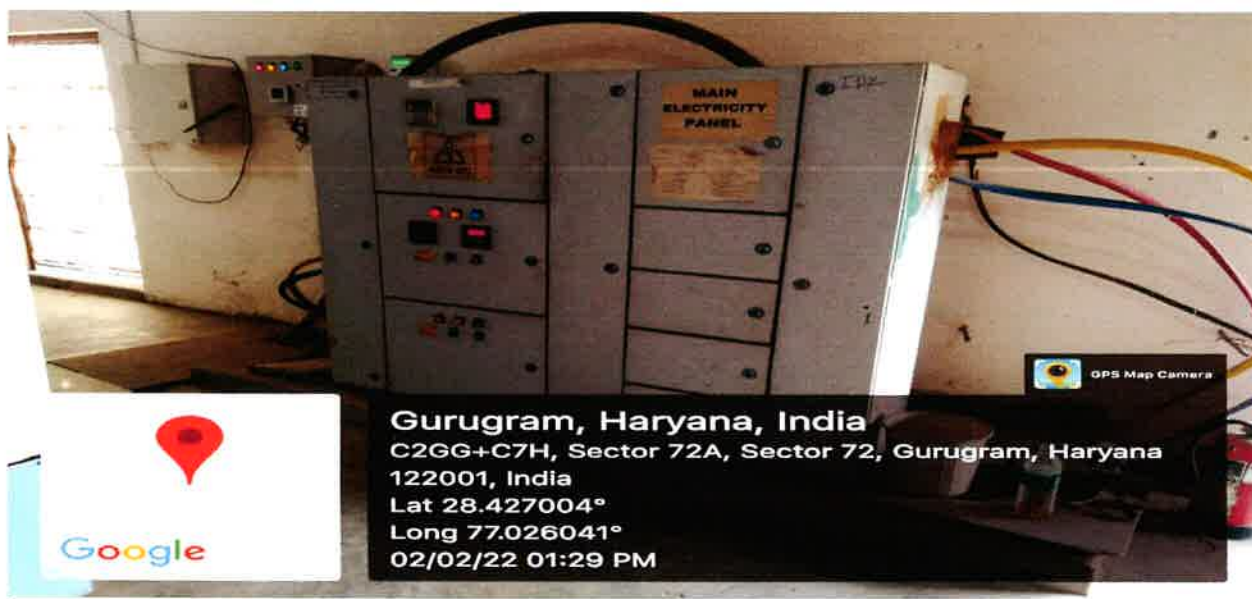
GENERATOR ROOM (Near Sports Ground) Annexure 4.1.1. (20)
