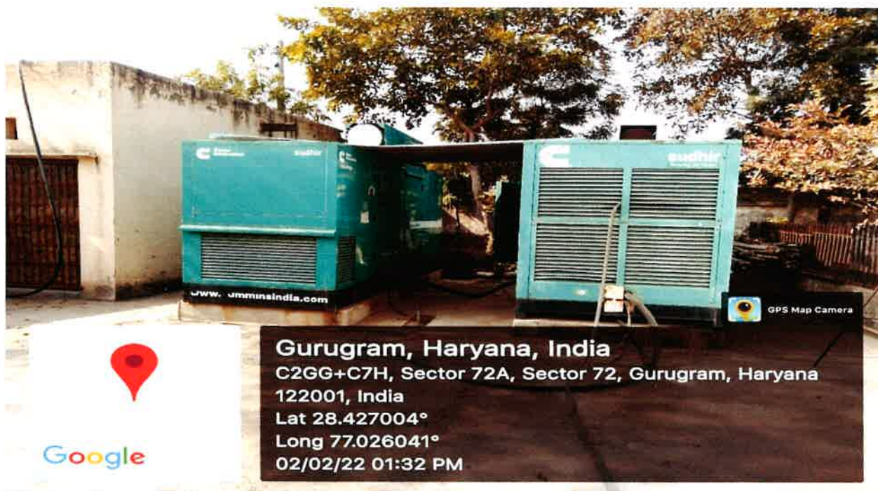
GENERATOR SET (Near Sports Ground) Annexure 4.1.1. (20)
