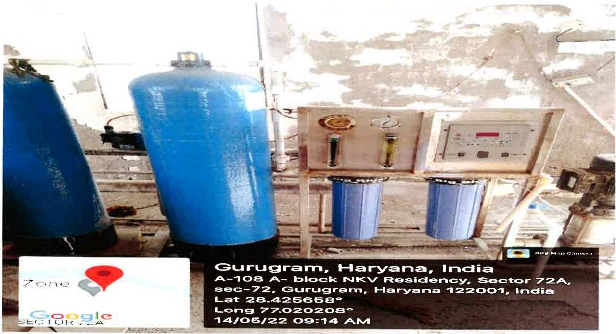
R.O PLANT FOR PURIFIED WATER (Roof Top-Block A and Block D )Annexure 4.1.1. (21)
